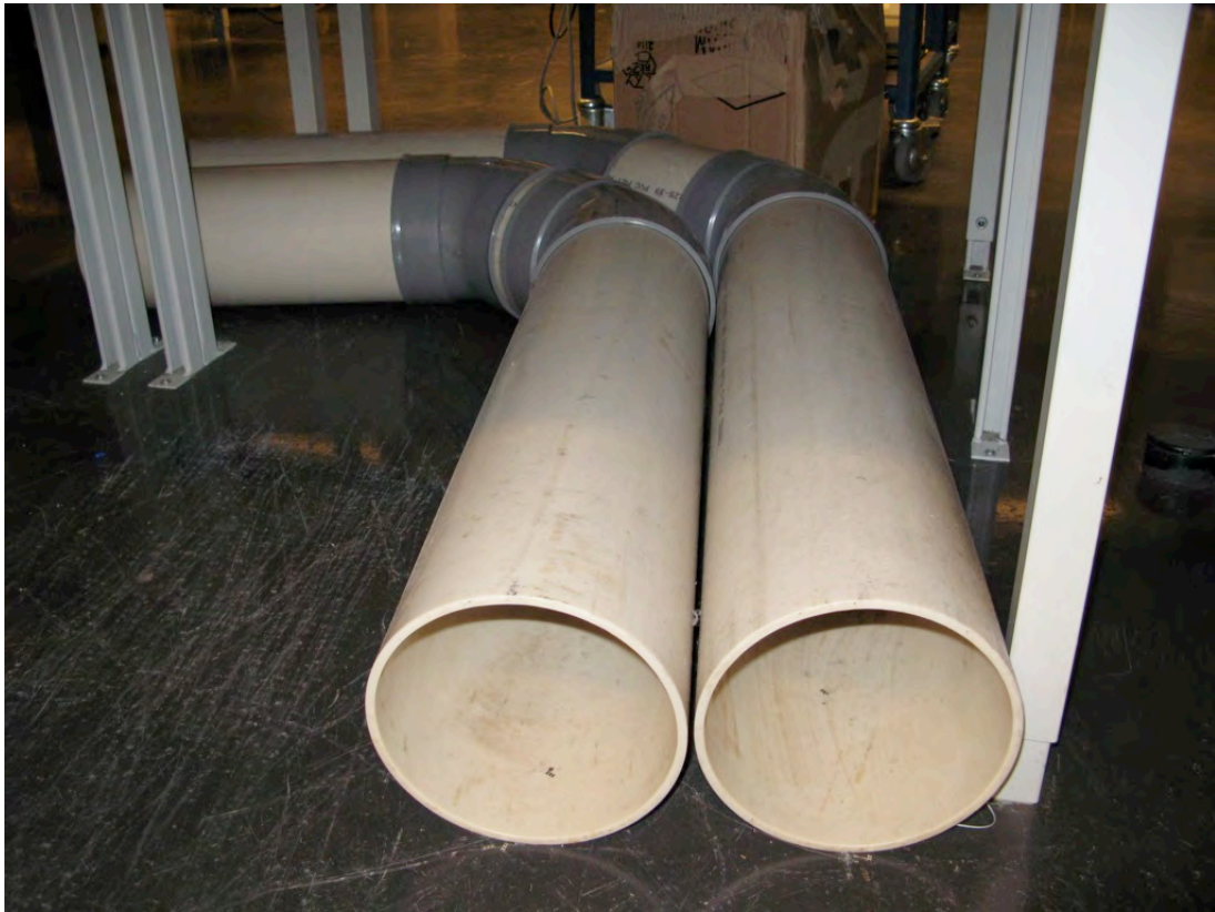
Figure 5.2-1: Example of the plastic tubes for the antenna cables as defined in the drawing above.
