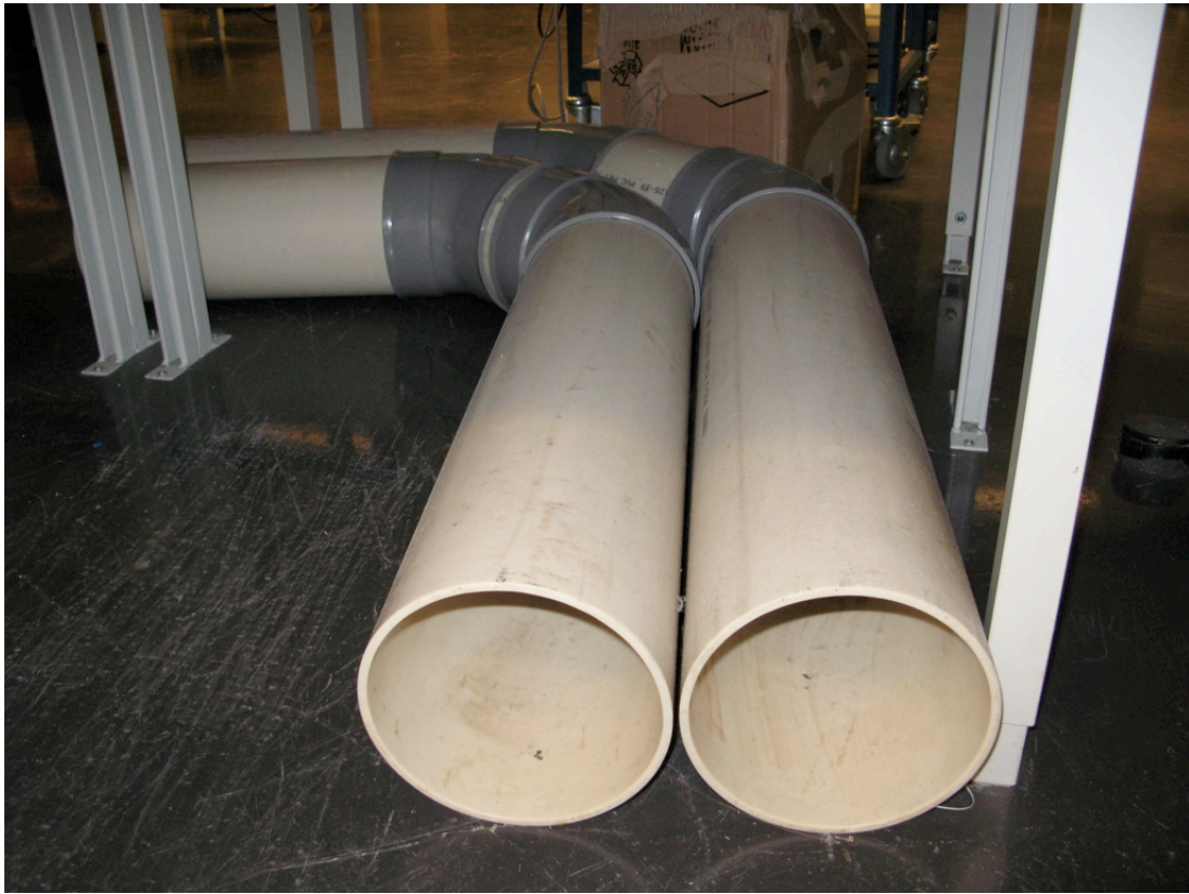
Figure 5.2-1: Example of the plastic tubes for the antenna cables as defined in the drawing above.
