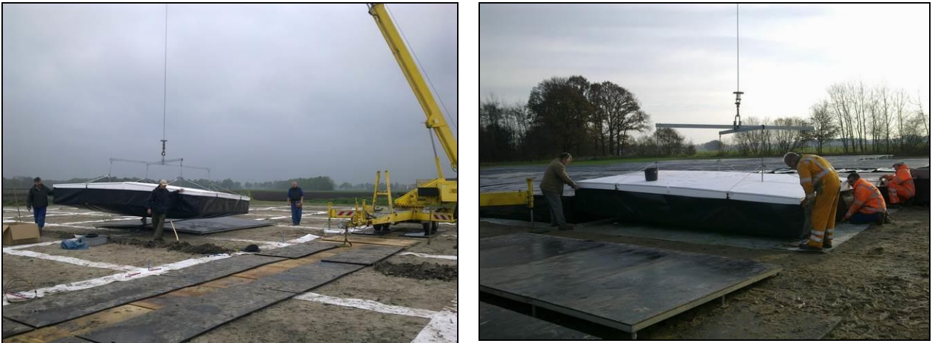
Positioning HBA tile (Note: POLFAR roll-out will not be executed in this manner)
