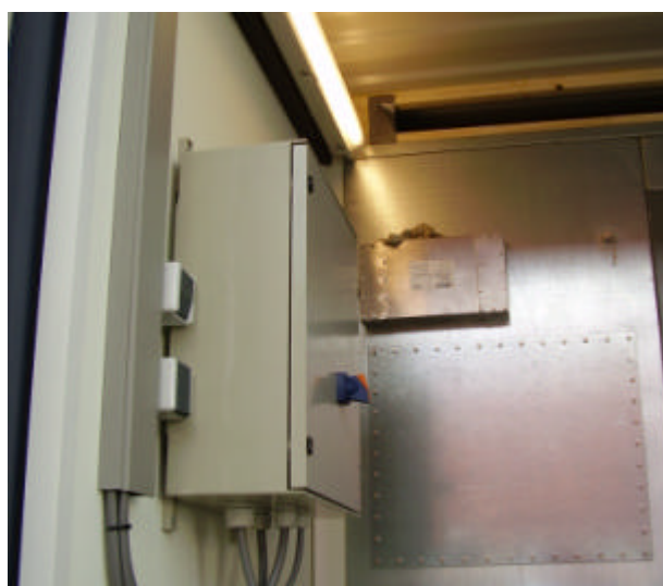
Overview of electrical installation in entrance section
